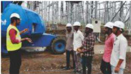
SPGVL 765/400KV Substation - Dhule
