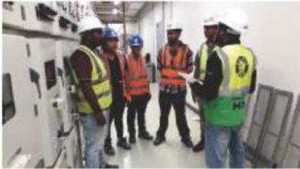
132/11kV Umm Al Hou1-2 Substation
