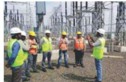
HERO SOLAR ENERGIES- SOUTH BUDH
