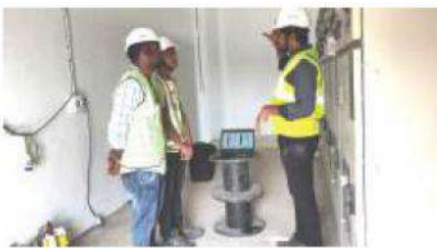
132KV Gaurav Project - Aurangabad
